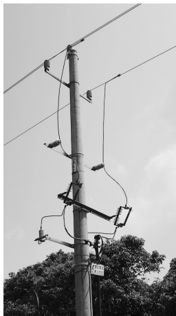
Figure 1.2 Conventional Railway Power Lines
